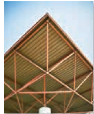
Typical roof-supporting space truss. Notice the use of ball-and-socket joints for the connections. (© Russell C. Hibbeler)
